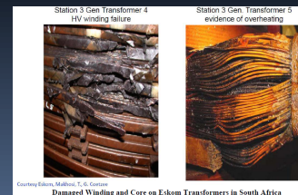
Damaged South African Transformers
