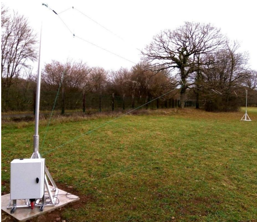
Figure 19: Transmission antenna in Dourbes, continuously transmitting at 4.59 MHz.
